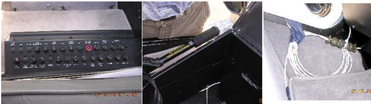
Figure B.2: Power Cable Routing: CB panel, under seat, cable dressing.
